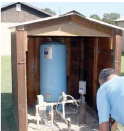
Home well water system
